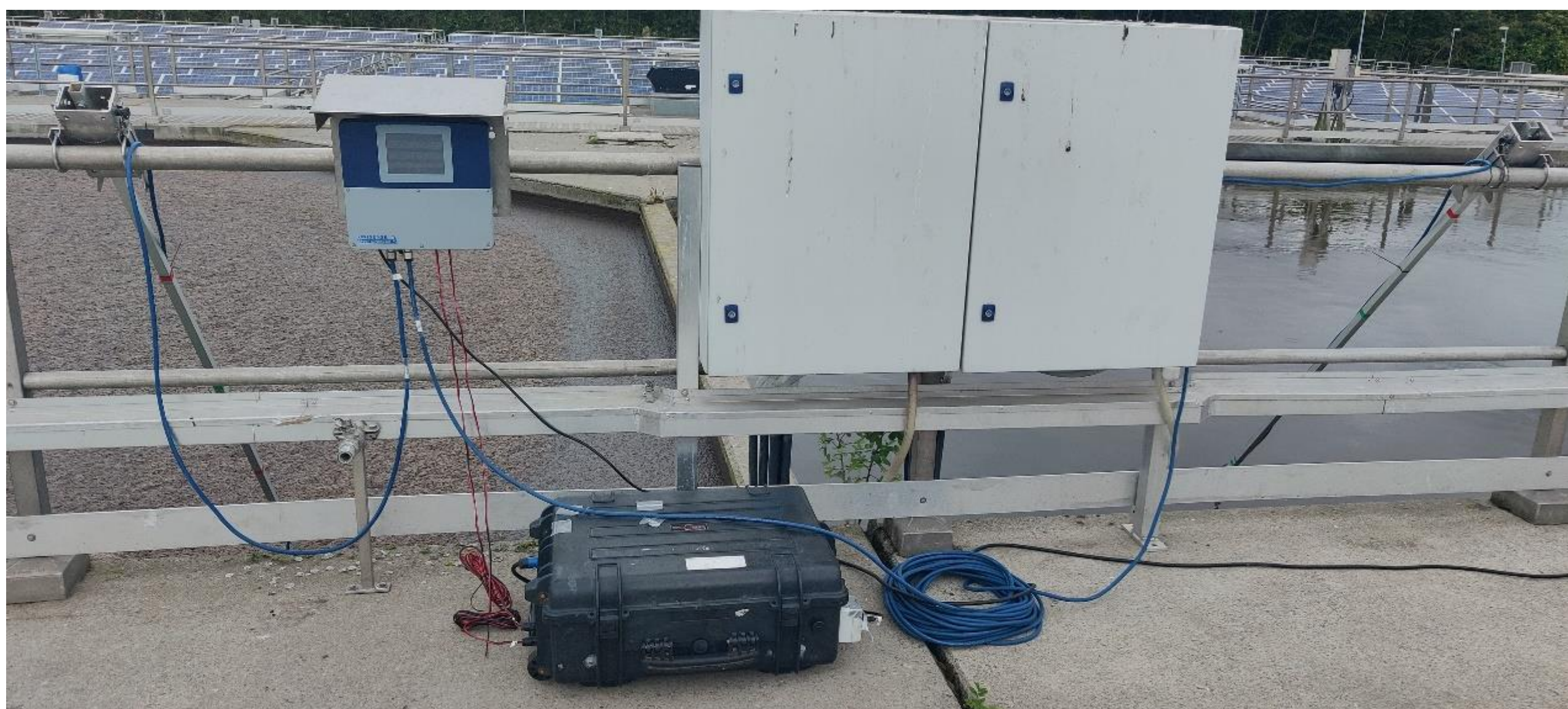
Figure 1 – Sensor controller box, monitoring suitcase and equipment for sensor mounting used during the N 2 O monitoring campaign.
