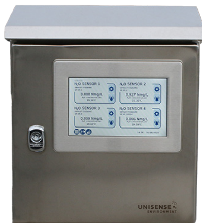
N 2 O Wastewater Operator Console
