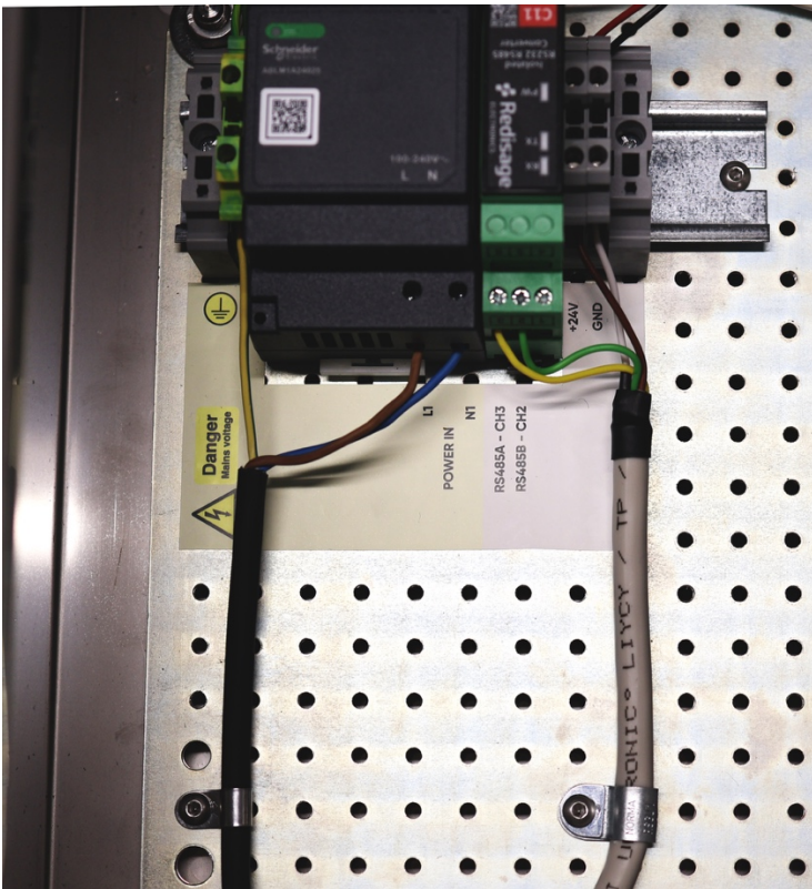
Picture 1: Cables inside the N 2 O Wastewater Operator Console (sample label). Note: The wire color coding shown is provided for reference and may not match the actual wiring.
